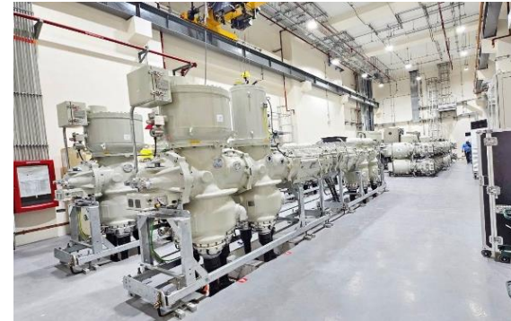
Development of Regalado 115 kV GIS Switching Station
