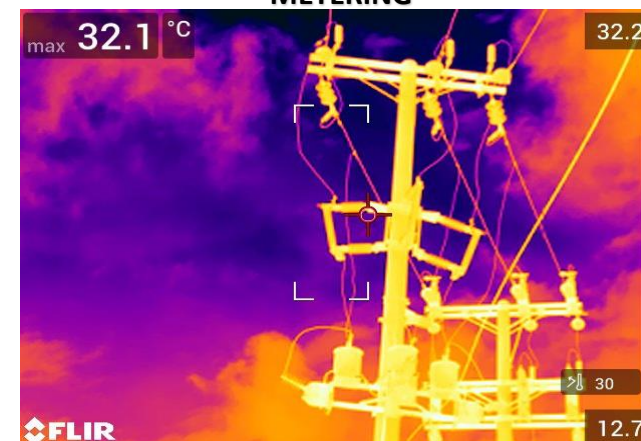
SCANNING PRIMARY METERING
