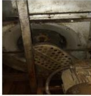
Photo No: 0037 Location: Hallway Caption: Fair Condition Fan Belt
