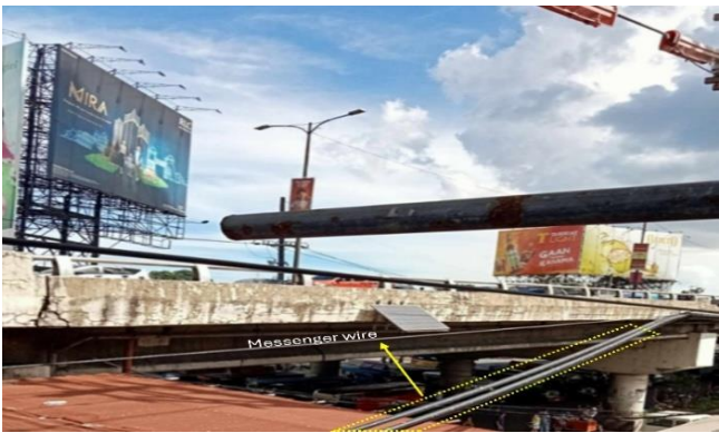
Figure 2. Example of a stolen spinning wire, causing the spun cables to sag as it has been detached from the messenger wire.
