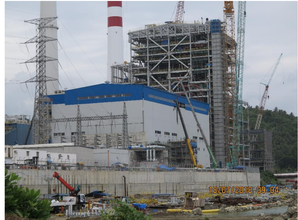
STG and Boiler
