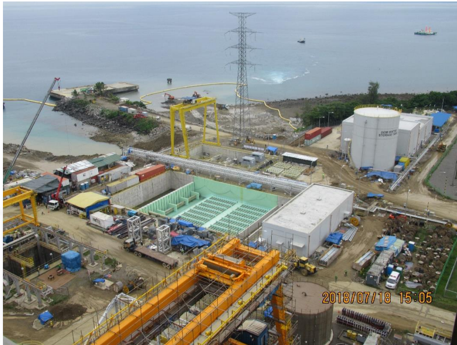
SWFGD Aeration Pond, Electrical Control Building and Intake Structure, Demin Water Tank & Water Treatment Area
