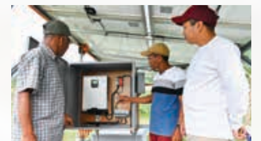
Aeta elders inspect a solar photovoltaic (PV) system installed by OMF in their community in Capas, Tarlac in partnership with Project Liwanag PH and Meralco's Corporate Business Group (CBG).
