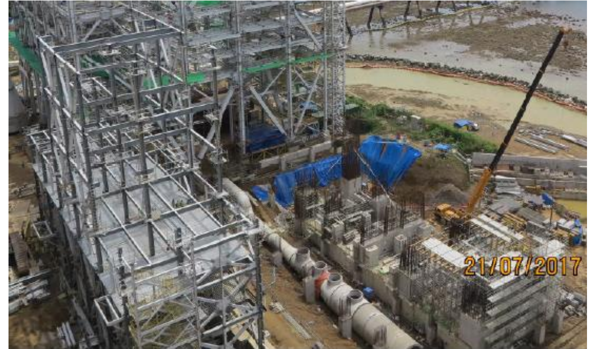
Control Building and STG Area
