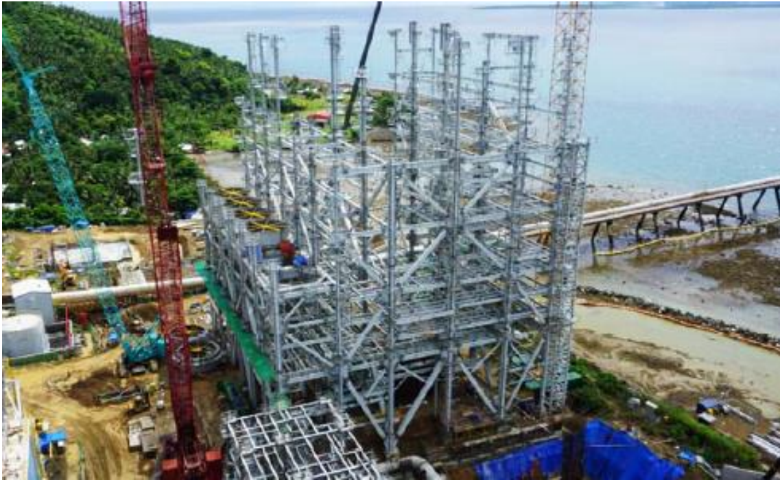
Pulverizer and Boiler Area
