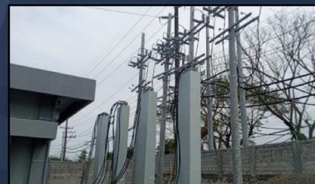
New Feeder Pedestals
