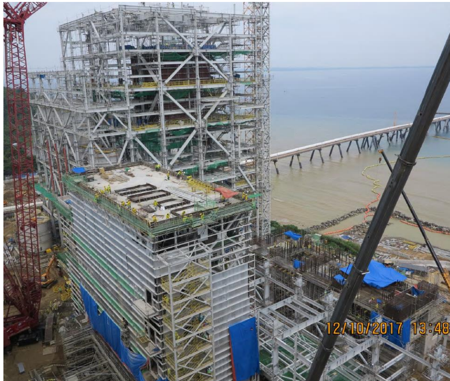
STG, Control Building, Boiler and Pulverizer Area
