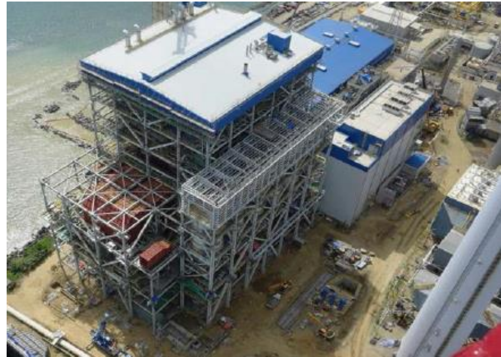
Boiler, Control Room and STG Buildings
