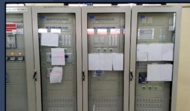
Protection & Control Panels
