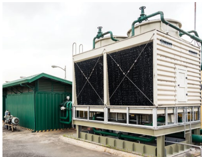
The chiller plant was installed in October 2014 on top of the Business Solutions Center at the Meralco Compound.
